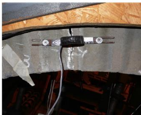
(b) Extrados crack C_{NA} .
