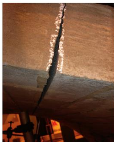
(a) Intrados crack C_{N1} .
